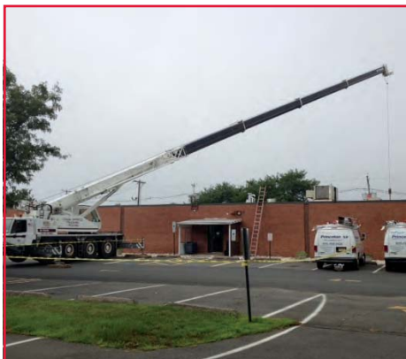
Our friends at Princeton Air installing new HVAC units at Clayton Center.
